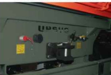
Hydraulic, pneumatic and electric connection to second trailer
